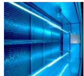
UV Lights - Coils
